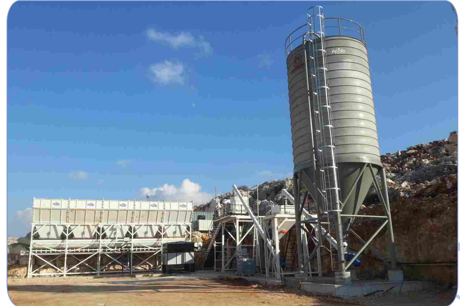
Apollo Dry Batching Plant : upto 120 m 3 /hr
